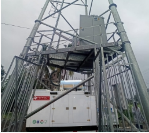
American Tower Company 15, 25 & 40 kVA x 324
