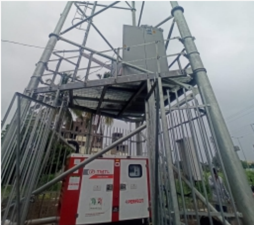
Telecom DG set with Internet Inside
