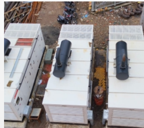
Data Centre Project 750 kVA x 40
