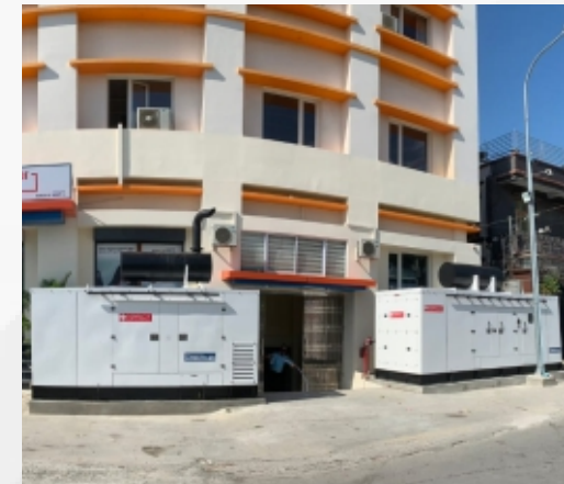
Hospital Project in Myanmar 400 kVA x 2
