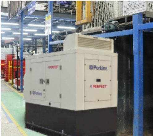
1000 Hours Long Maintenance DG set
