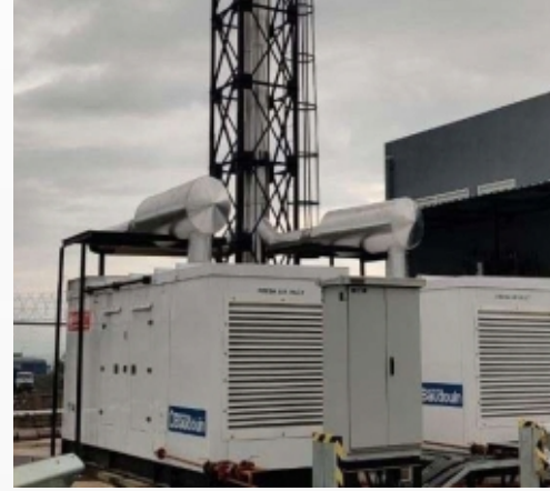
Amazon Project 400 kVA x 2
