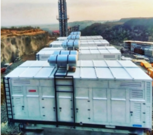
3.3 kV / 6.6 kV / 11 kV High voltage DG set
