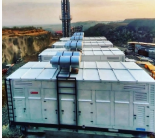
High Speed Roadway Project 2000 kVA x 8
