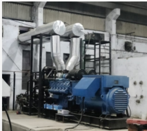
HDPE Manufacturing Units 1250 kVA x 2 & 1010 kVA x 2
