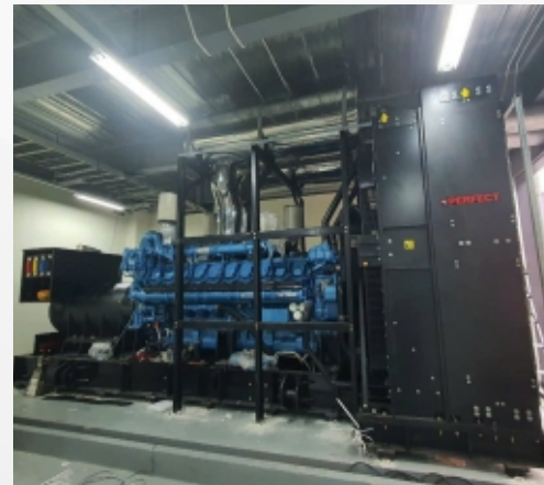
Industrial Unit in Vietnam 2500 kVA x 1
